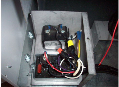
Typical igniton board.
